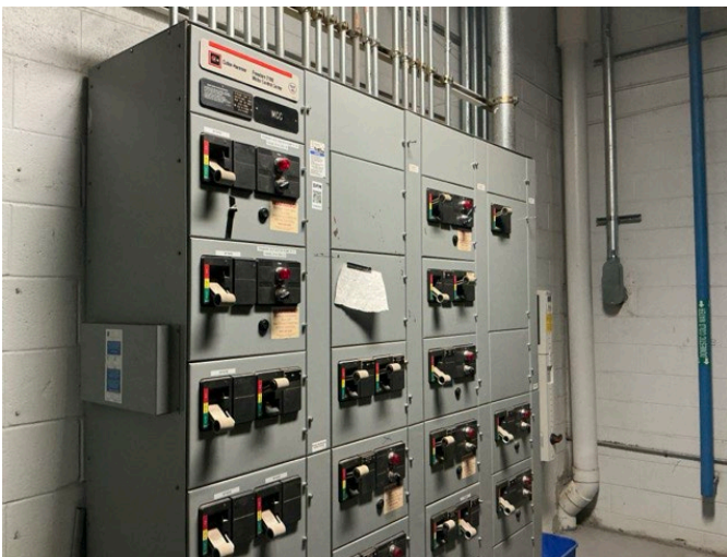
27 - MOTOR CONTROL CENTER
